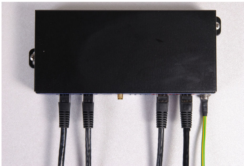
Figure 5-12 PTP-SYNC mounted on a wall
